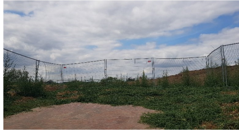
20b. Footpath 728 from the edge of the Peake Way site with the play area/ landscaping under construction
