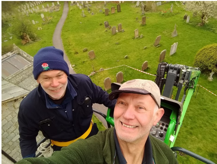
Carrying out repairs to the flag pole on the church tower. Top left: the 'cherry picker' in action. Top right: the Union Flag proudly flying from the repaired flag pole. Bottom: two of our four intrepid steeple jacks, Joss and Paul.
