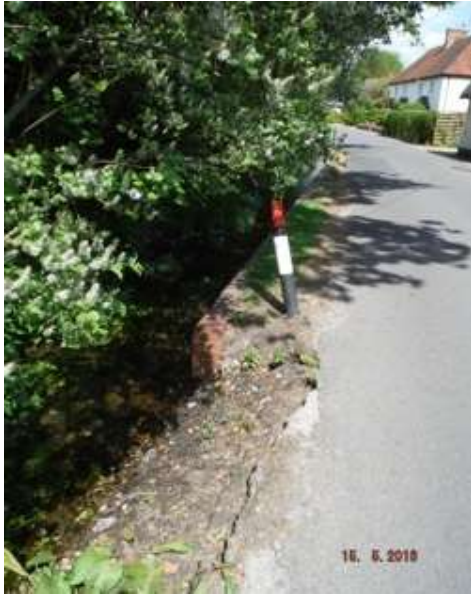
Figure 26 – Village Street crumbling in to the Winterbourne.
