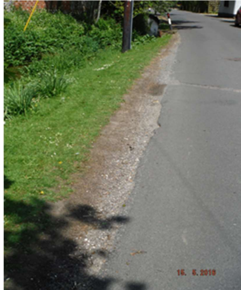
Figure 27 – Winterbourne verge and road edge eroded by vehicle tyres.
