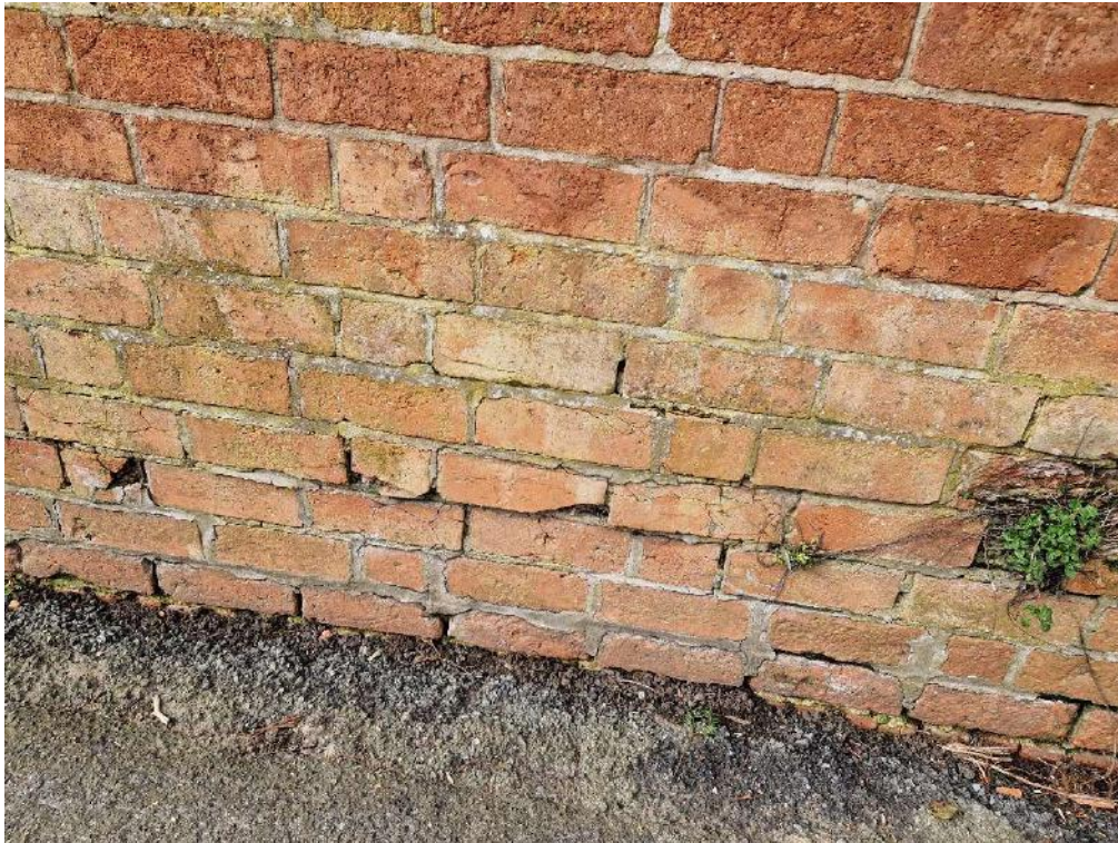
Photograph No. 25 – East – Sheared Wall at Low Level
