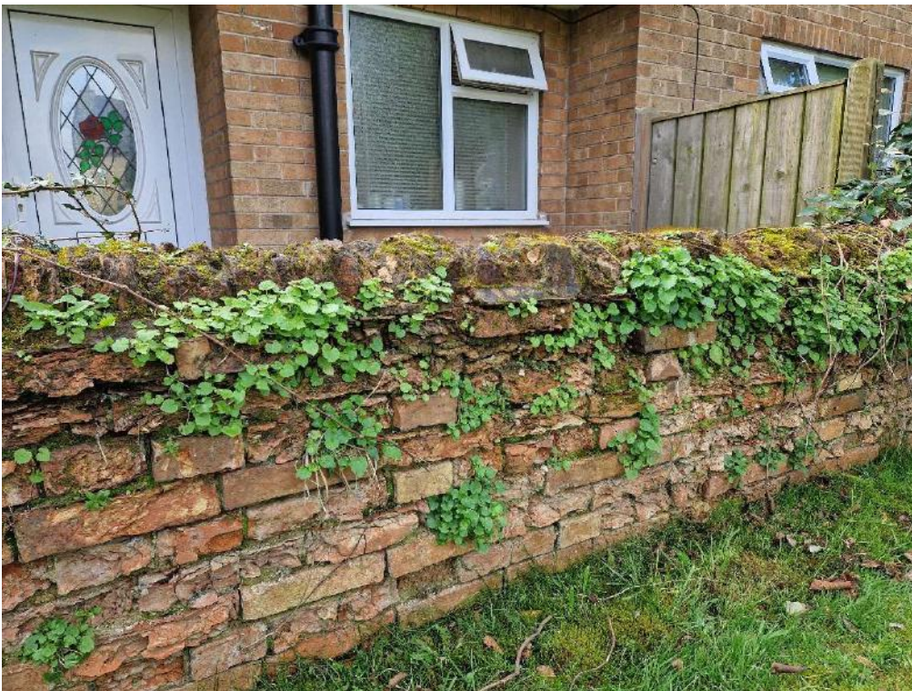
Photograph No. 28 – South – Deteriorated Masonry Throughout Wall
