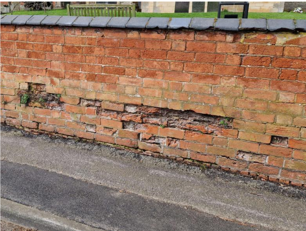
Photograph No. 24 – East – Deteriorated Masonry at Low Level
