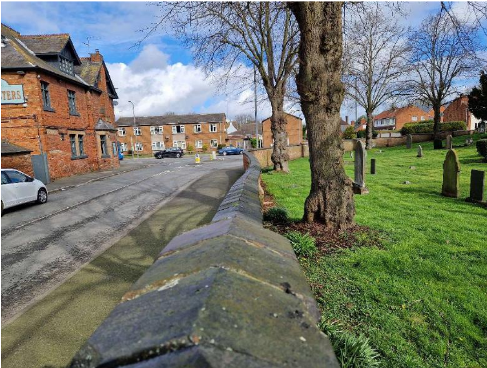
Photograph No. 16 – West – Deflection to Span 7
