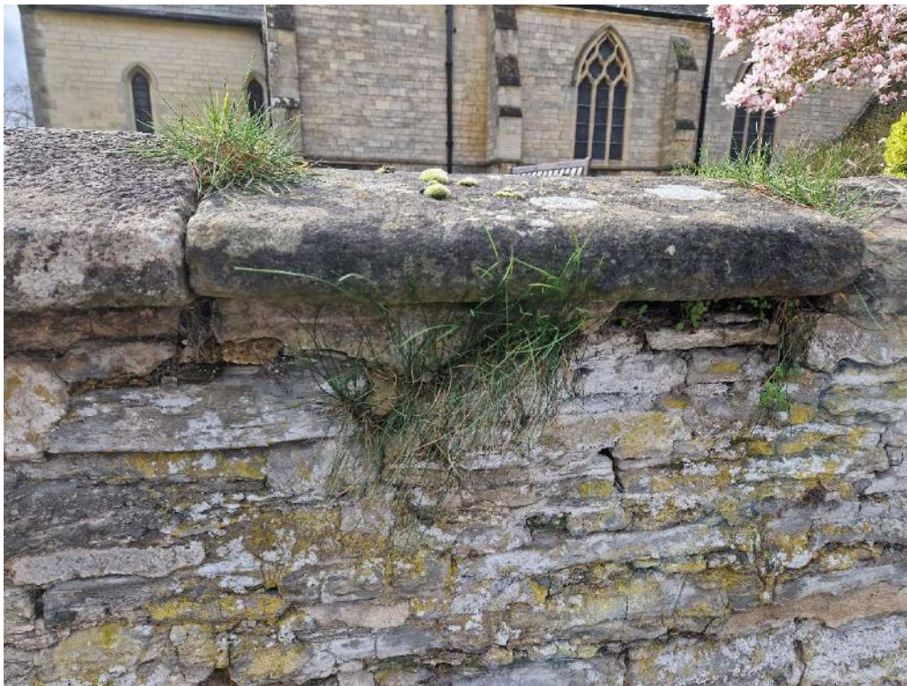
Photograph No. 22 – North – Foliage Growth on Wall
