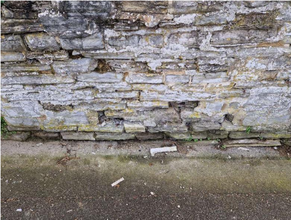
Photograph No. 23 – North – General Areas of Deterioration Due to Age
