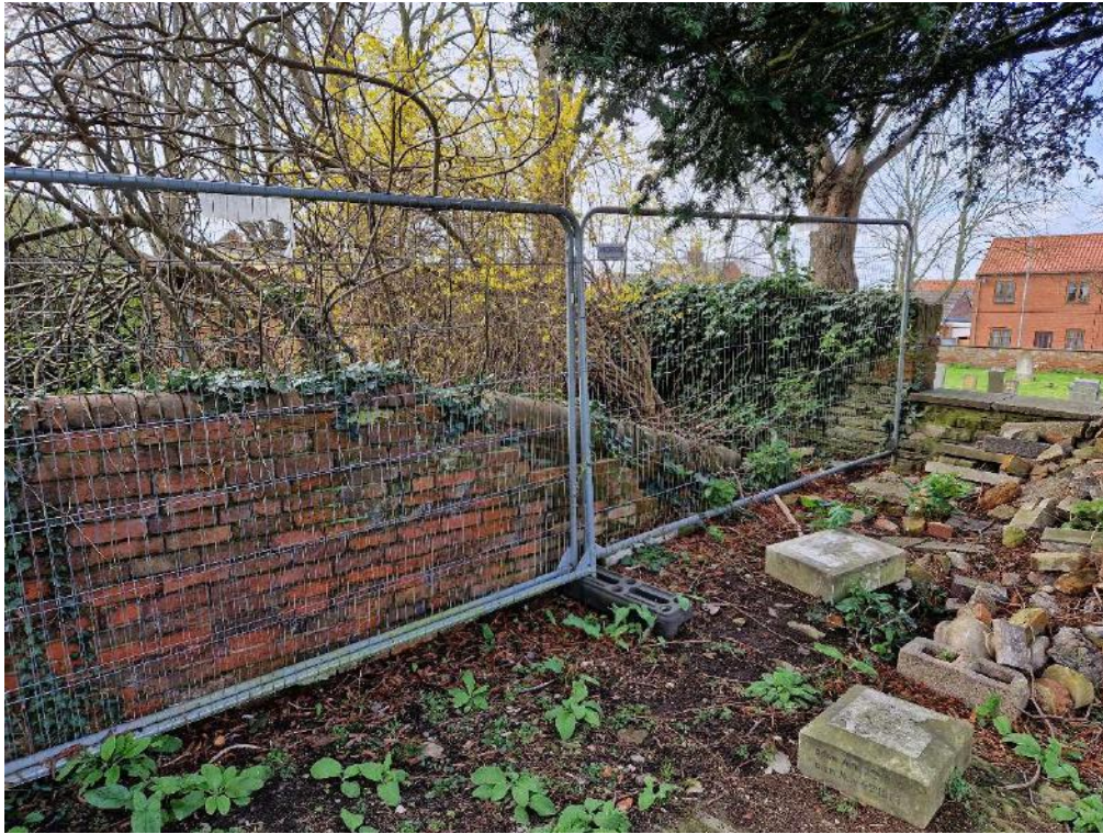
Photograph No. 29 – South – Collapsed Section of Wall
