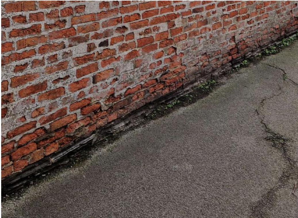
Photograph No. 11 – West – Scour at Base of Wall and Blue Lias Used as Base
