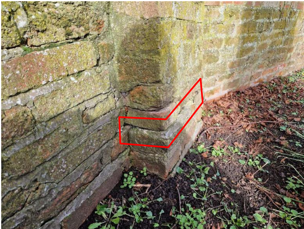
Photograph No. 18 – West – Deteriorated Pier with Lateral Movement at Base
