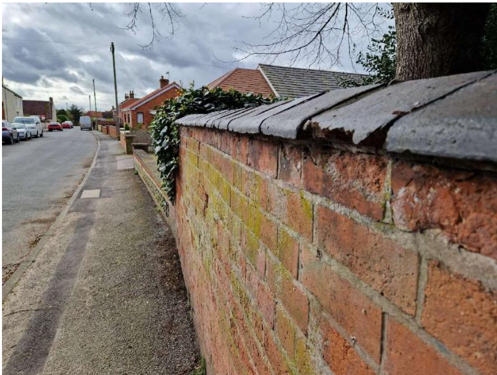
Photograph No. 26 – East – Minor Concave Shape to Wall at Southeast Corner
