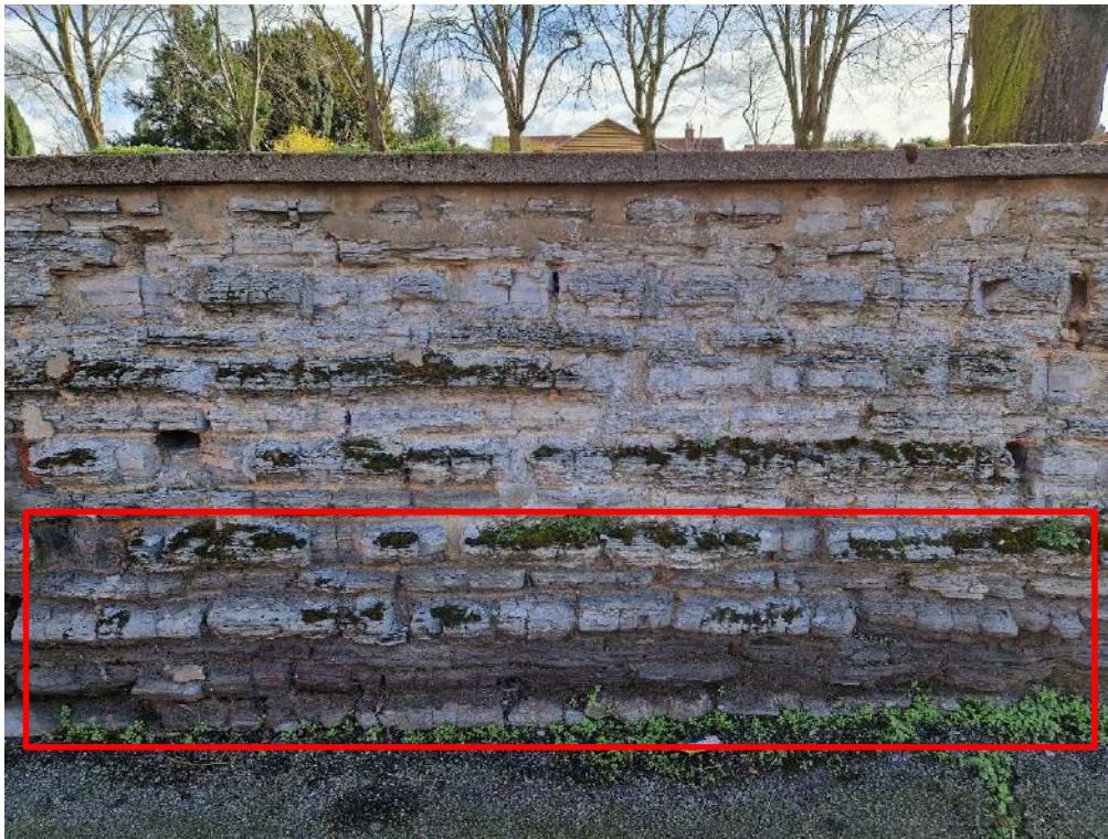
Photograph No. 5 – West – Noticeable Change in Colour at Low Level
