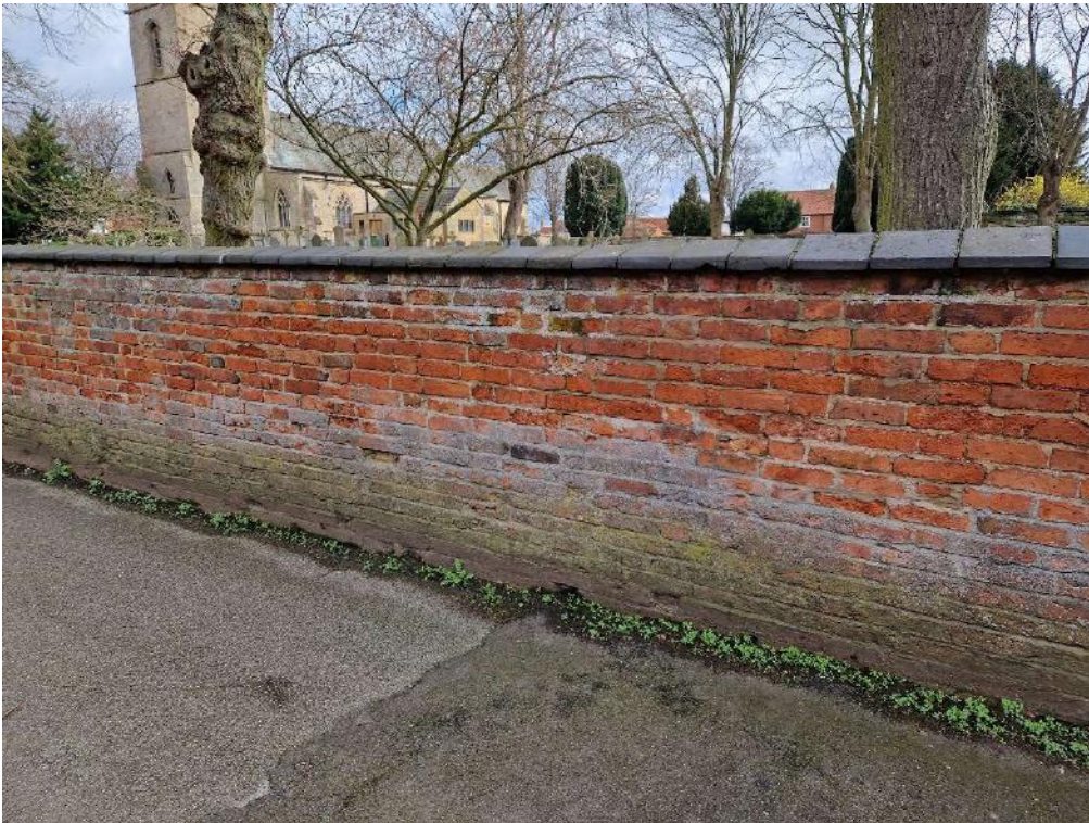
Photograph No. 14 – West – General Condition of Wall Section and Efflorescence to Lower Half
