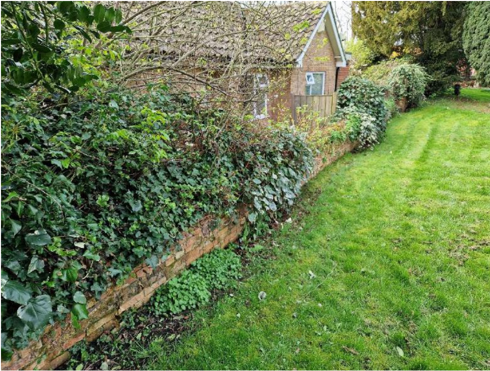
Photograph No. 27 – South – Foliage Growth Along Wall
