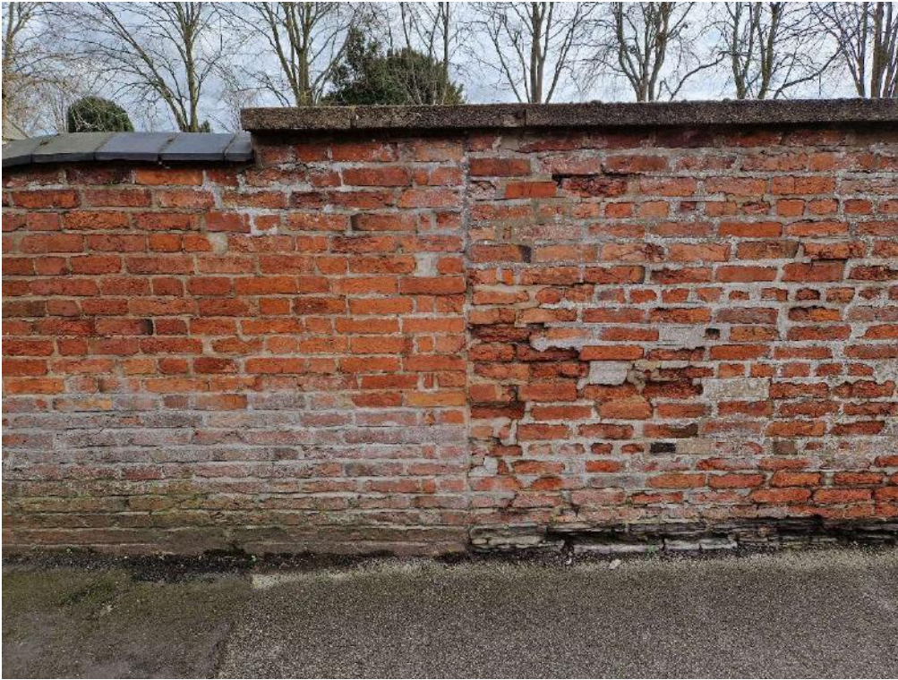
Photograph No. 13 – West – Interface Between Span 5 and 6
