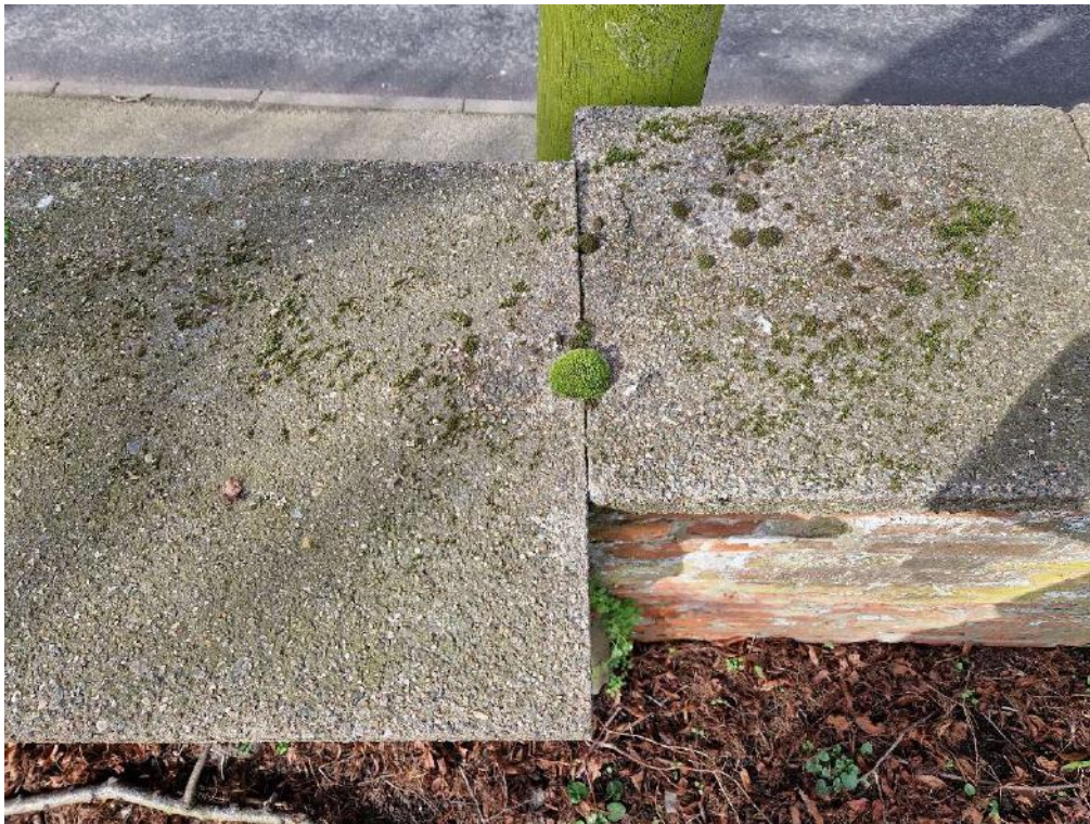
Photograph No. 9 – West – Misaligned Coping Stone Between Span 4 and 5
