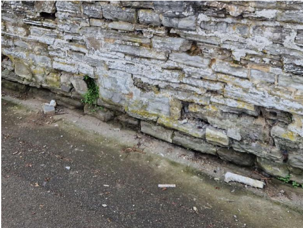
Photograph No. 21 – North – Scour at Base of Wall
