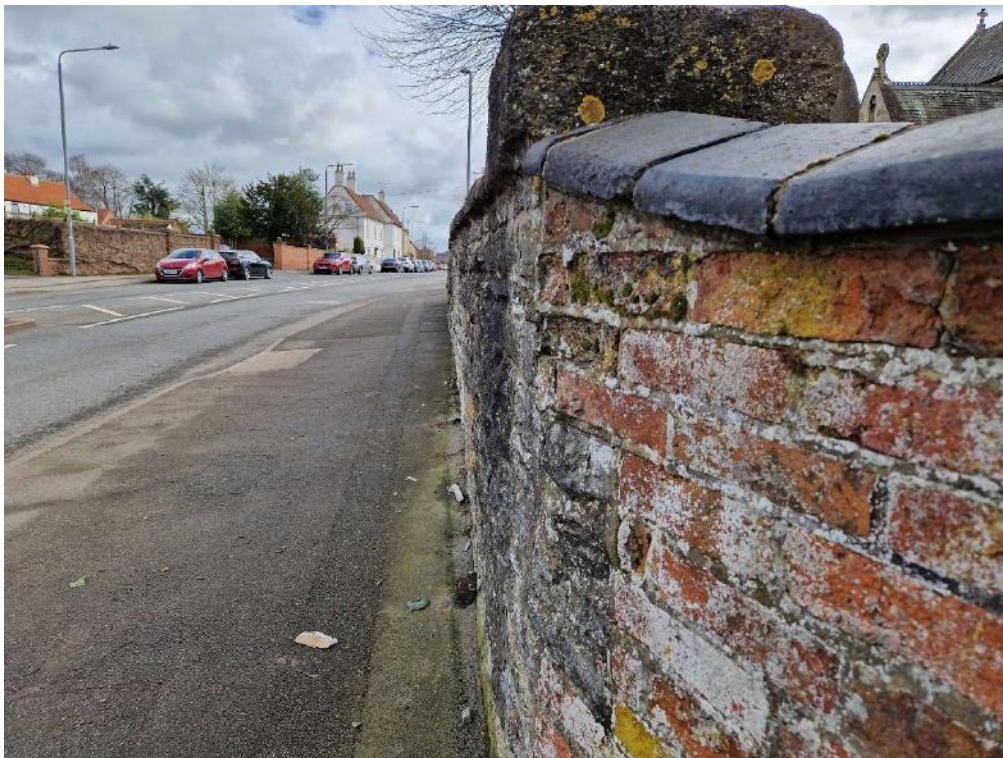
Photograph No. 20 – North – Observed Undulations and Minor Lean
