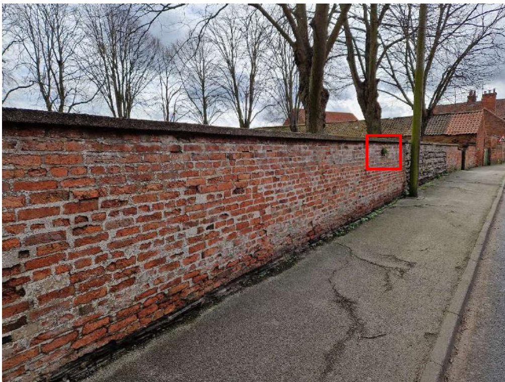
Photograph No. 10 – West – Span 5, Highlighted Foliage Growth
