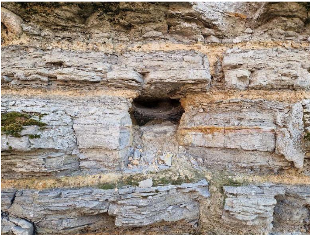
Photograph No. 6 – West – Areas of Missing Masonry and Mortar
