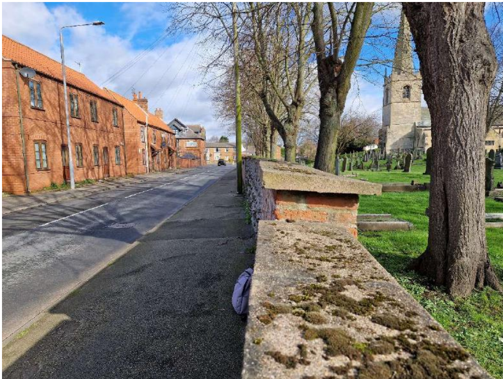
Photograph No. 8 – West – General View of Lean to Front Face of Wall
