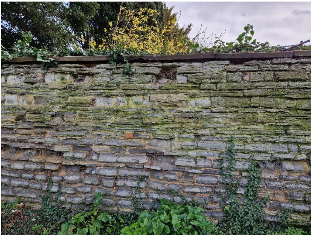
Photograph No. 30 – South – Deteriorated Masonry/Mortar Along Wall Length
