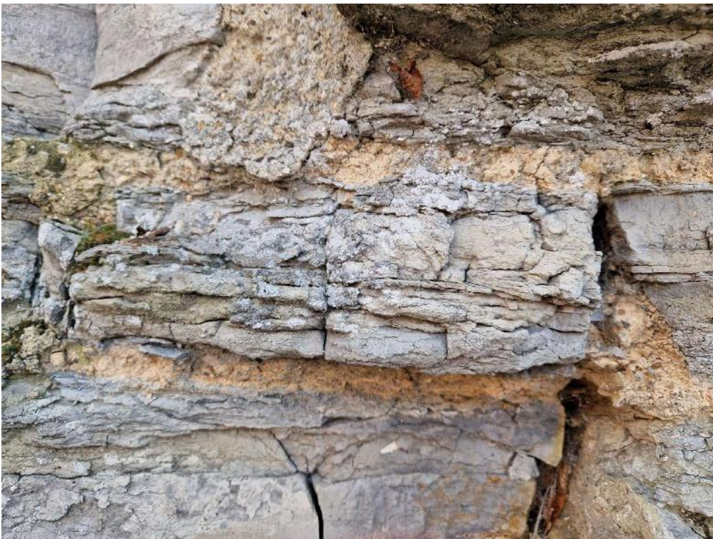
Photograph No. 4 – West – Heavily Deteriorated Masonry and Mortar
