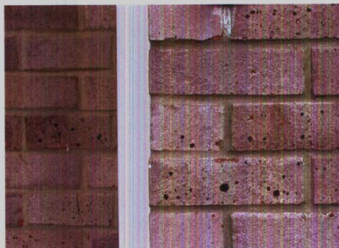
Pastel coloured sand faced common bricks are inappropriate in a flint and brick area
