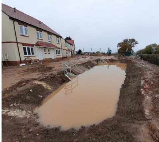
Left: balancing pond at Carrots Farm, North Petherton. Right: headwall pipe measuring at Wayside Farm, Castle Cary.
