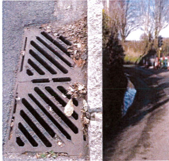
No action required: Intervention level not met
