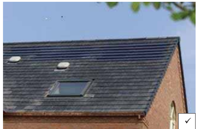
Solar tiles which merge almost imperceptibly with the existing roof tiles
