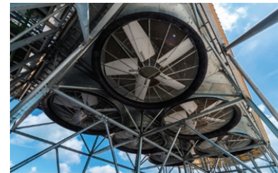
Extractor fans at Ardley
