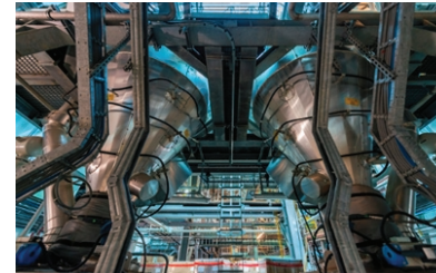
Turbines at Ardley
